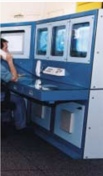
Colliery Control Room
